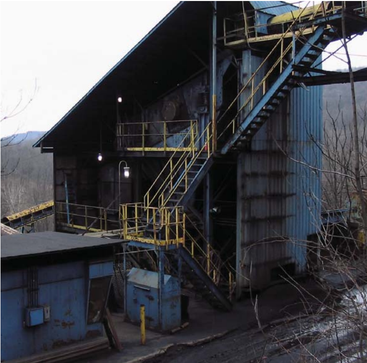
Built in the 1970s, Beechwood Coal Co.'s Lonaconing tipple has a raw feed capacity of up to 600 tph.
